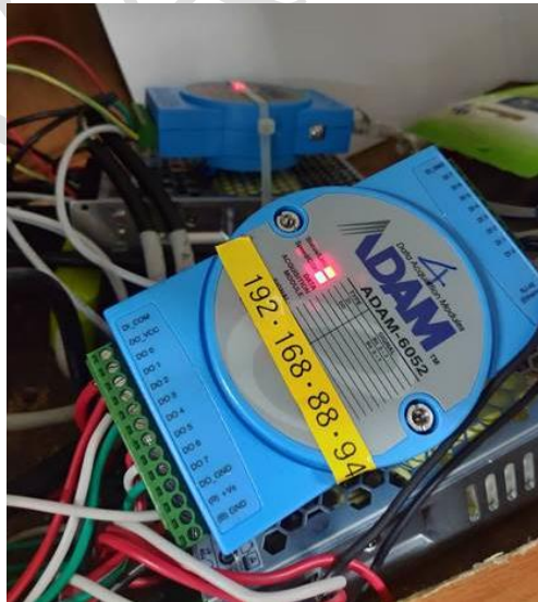
Figure 1 Improper way to install and use ADAM module at the field
